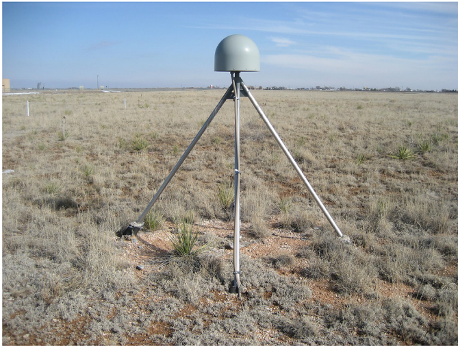
Fig. 1. Photograph of GPS site at P038 in Portales, New Mexico ( http://www.unavco.org ). The antenna is under the hemispherical radome. The receiver is stored in a nearby equipment box. The antenna phase center at this site is approximately 2 meters above the soil surface.
